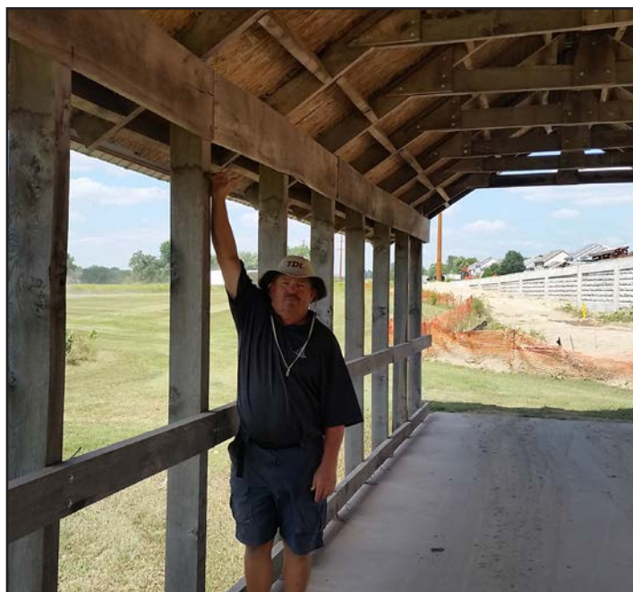
Photo: Water Line on Bridge.
